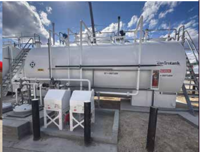
Bulk fuel storage systems, installed and serviced.
